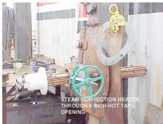
Figure JL-2. Photograph of the heat exchanger unit inserted through the 6-inch hot tap (Photograph courtesy of PCCI, Inc.).
